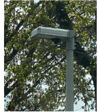
Luminaire LED routier (zagha)
